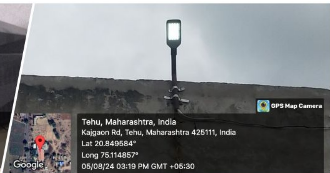
Tehu, Maharashtra, India Kajgaon Rd, Tehu, Maharashtra 425111, India Lat 20.849514° Long 75.114925° 05/08/24 03:16 PM GMT +05:30
